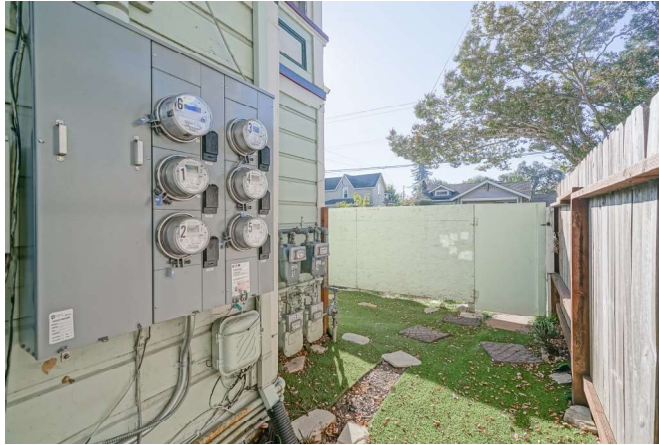
Updated electrical panel
