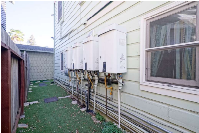
On demand hot water heaters
